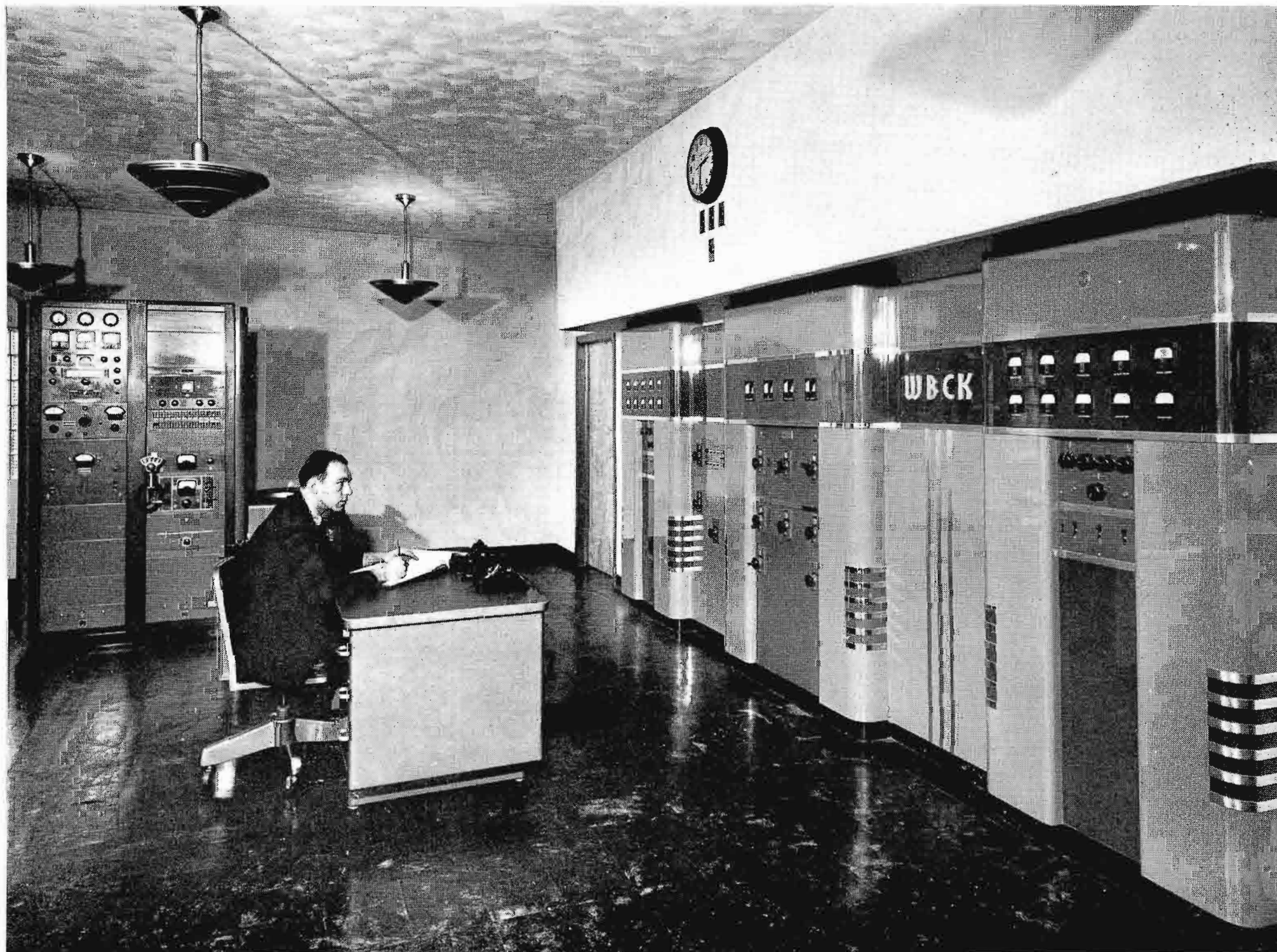
FIG. 1. (below). WBCK's 1 KW transmitter room view showing how phasing equipment is located between the 250-watt exciter and 1 KW amplifier cabinets. Chief Engineer, A. J. Geranis is at transmitter control desk. At far left are test and audio input racks.
